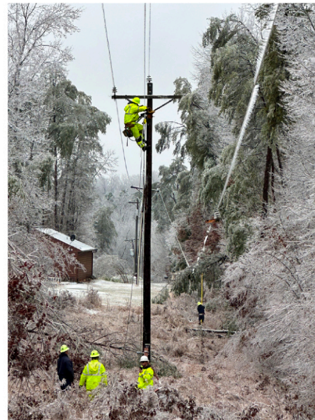
(Above) Substation crews repair cold-related equipment failure in Goose Creek. Overall, the co-op’s system performed well under heavy strain caused by Winter Storm Enzo.
