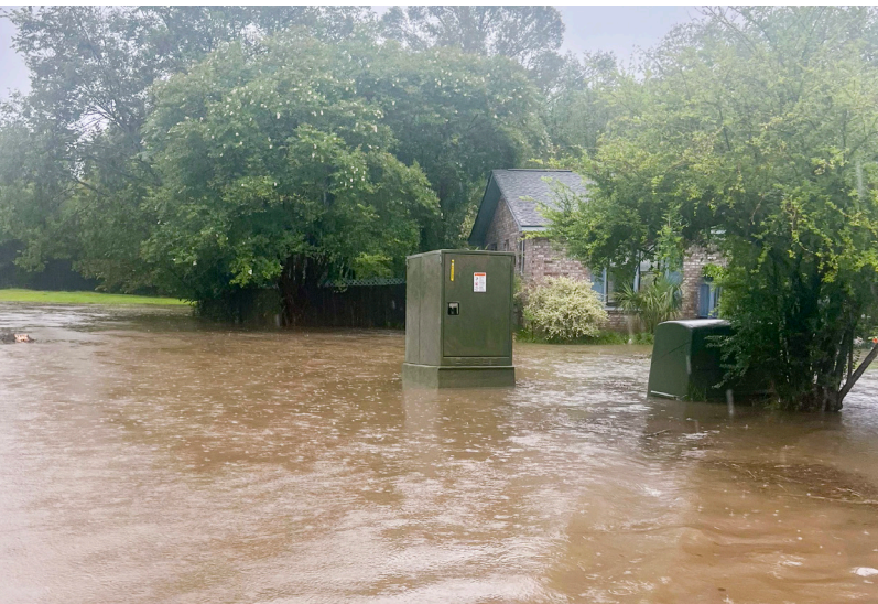
Berkeley stationed crews to monitor flood levels threatening underground equipment in College Park Estates,
