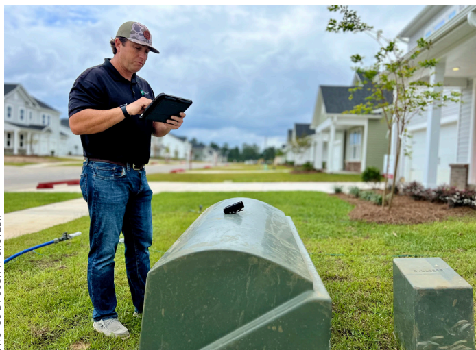
In the field, Jason Trussell and his team can easily update new equipment data, like this junction box in a recently built Goose Creek subdivision, using an iPad and an GPS location device.
