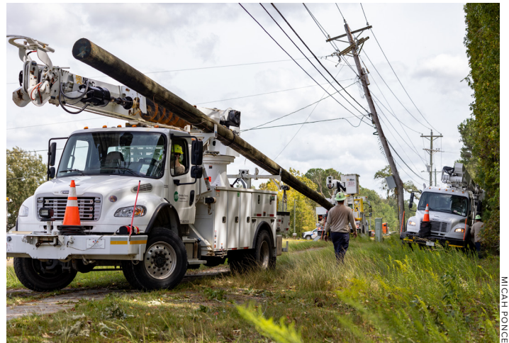
Hurricane Helene left broken poles across Berkeley's territory, including two on Liberty Hall Road in Goose Creek which shut down traffic for hours.
