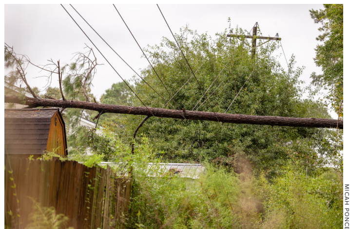
Fallen trees, like this one off College Park Road, were responsible for over 20 broken poles system wide. Each broken pole takes a four-man crew approximately two hours to replace under ideal conditions.
